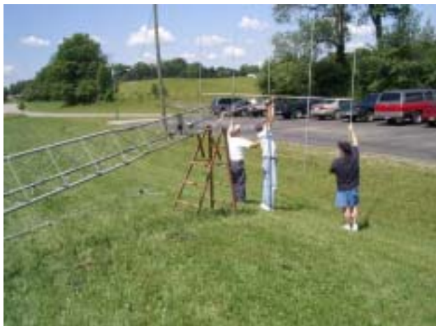
Assembling the 2, 6 meter array are Jim (l-r) WA8GXM Dan N8DZM and Scott N3JJT.
