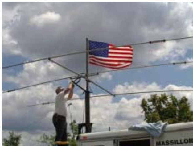
While 'Old Glory' flies in the breeze, Jim WA8GXM does the final "tune up" on the triband & dipole on top of the "rocket launcher" on front of the E-Com trailer.
