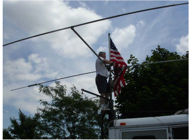
Now it's Jim's turn to finish the installation of the 3 element beam antenna for the phone station on the E-Com
